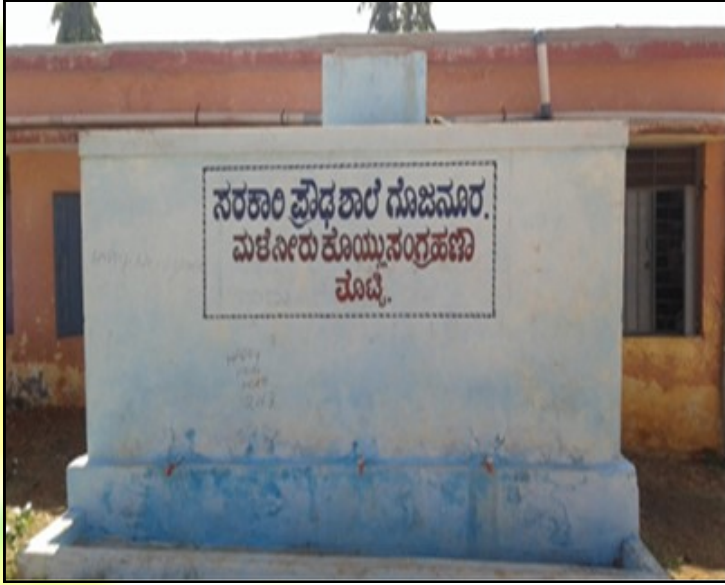
Rain water Harvesting Unit
